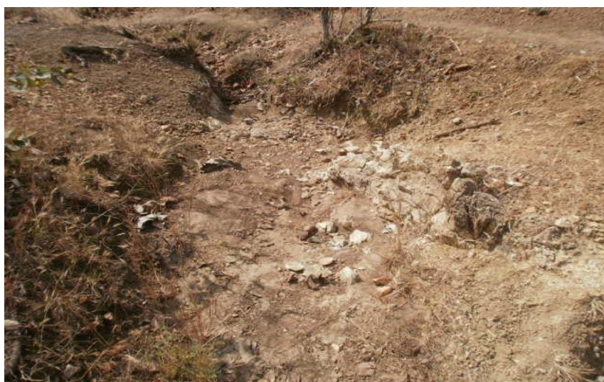
Plate V. Development of erosion channel arising from mining activity.
